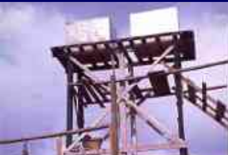
Water storage tanks
