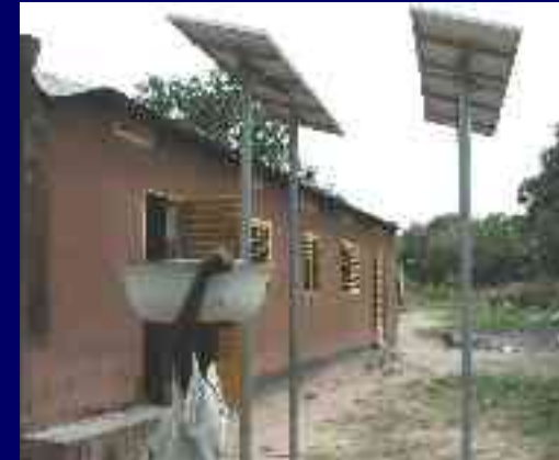
Solar power for a clinic
