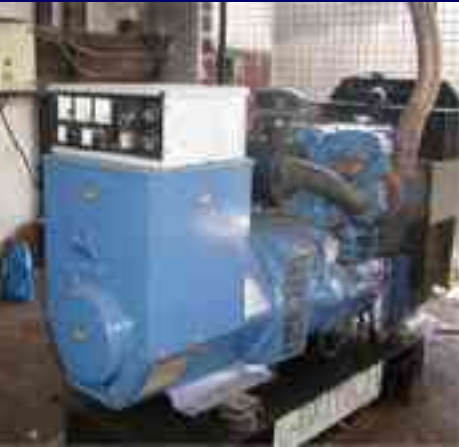
Diesel power plant
